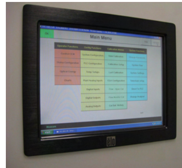
Touch screen system interface
