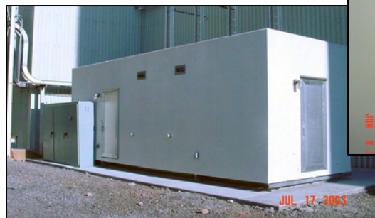
Successful CEMS Installation
